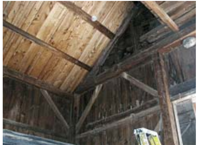
The framework of the barn provided important clues as to its age.
