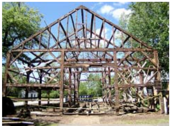
The frame of the barn was held together by approximately 250 oaks pins about an inch in diameter.
